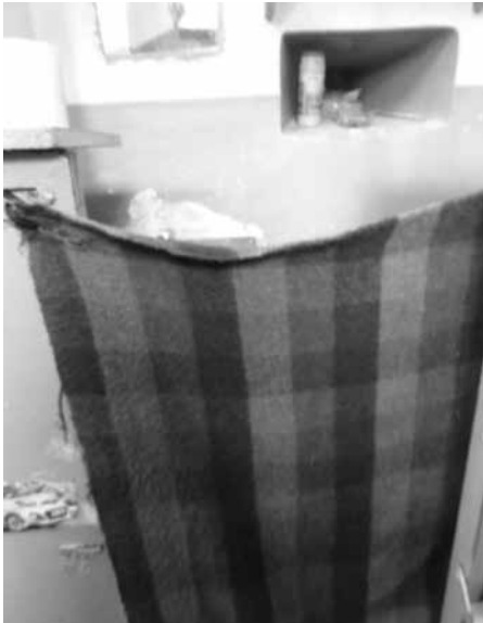
Toilet with a blanket instead of the door in the residential cell of the Prison in Racibórz
