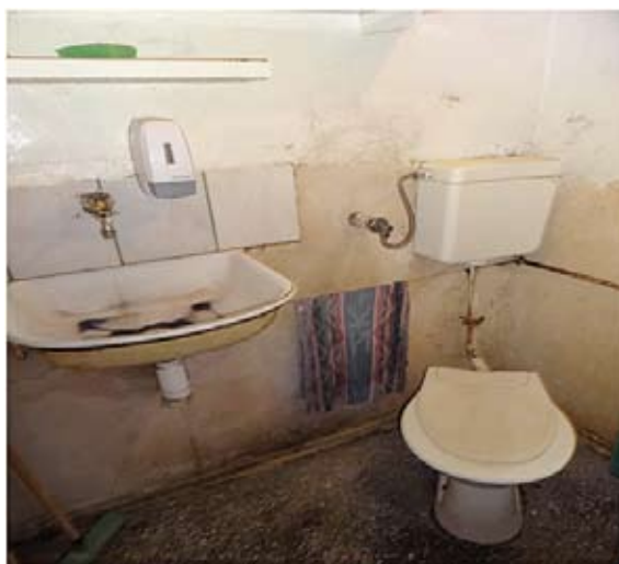
Prison in Wołów – sanitary facilities in one of the cell
