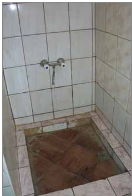
Sanitary facilities in the Prison in Uherce Mineralne
